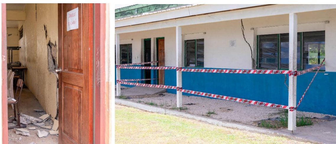
Image 2: Damage in schools on Efate after the 17 December 2025 earthquake.
